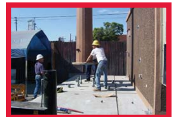
Installation of antennas, wave-guides, and equipment begun prior to end of day.
